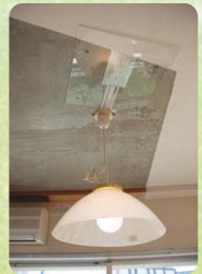
Wiring in tape-type cable
